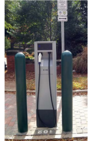
Photo 2. Pedestal-mounted EVSE installed by the City of Raleigh, N.C., for free public use. Photo from Kathy Boyer, NREL 18520
